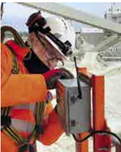
Installation des Gateways
